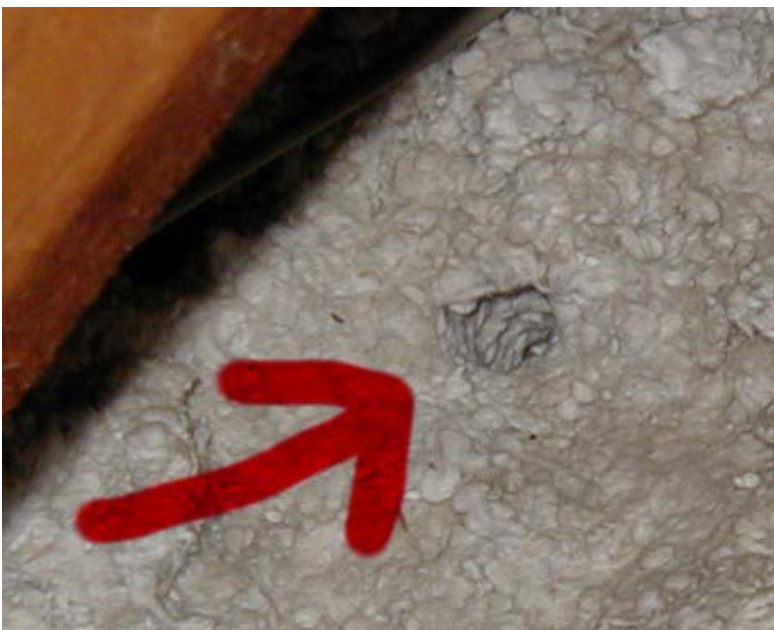
Mouse holes in attic insulation.
