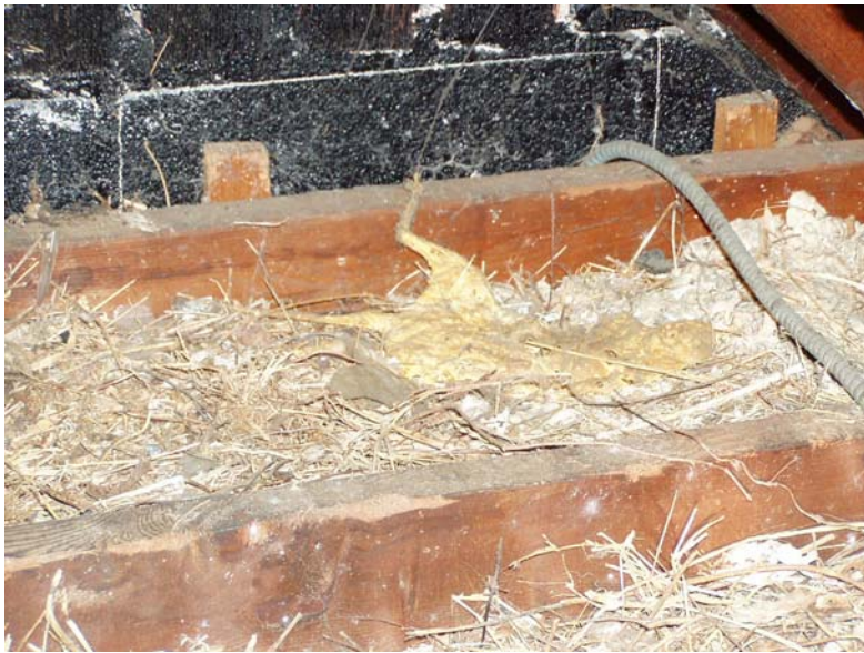
Remains of squirrel in attic floor. This house must have stunk for a while.
