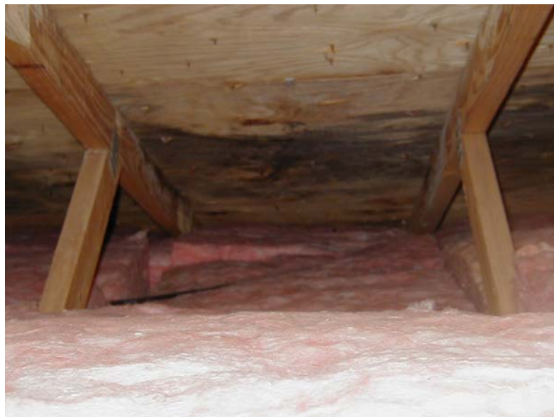
Condensation problem in attic. Some mold growth. (Unsafe)
