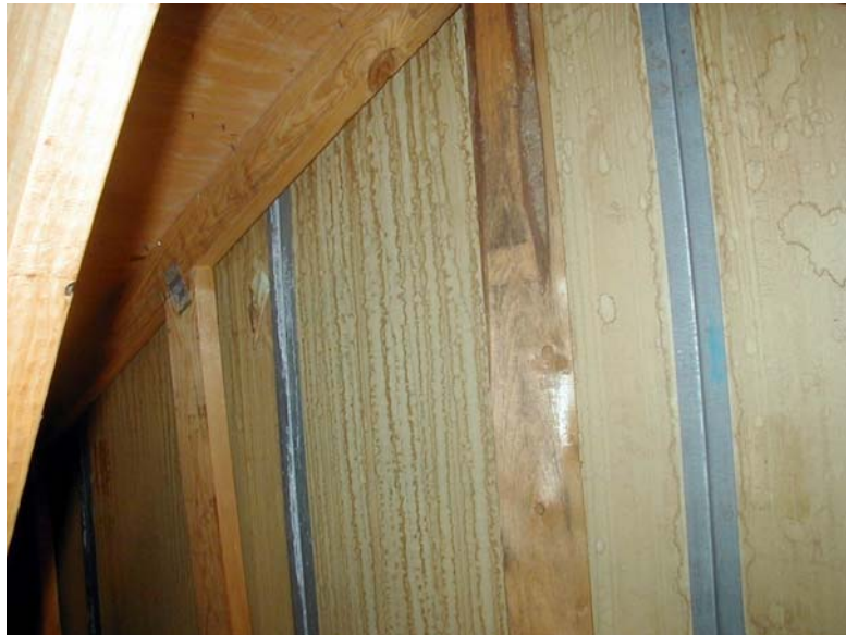
Leak stains on attic side walls, due to leaking step flashing.
