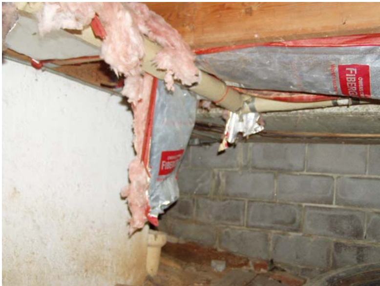
Insulation installed up side down. Insulation missing and falling.
