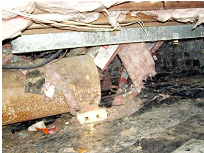
Abandoned oil tank needs to be removed. Falling insulation.
