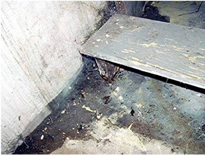
Rot damage to stair carriage, due to extensive water entry.
