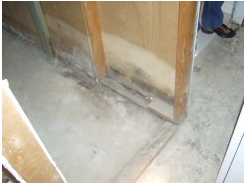
Mold growth on basement walls. (Unsafe)
