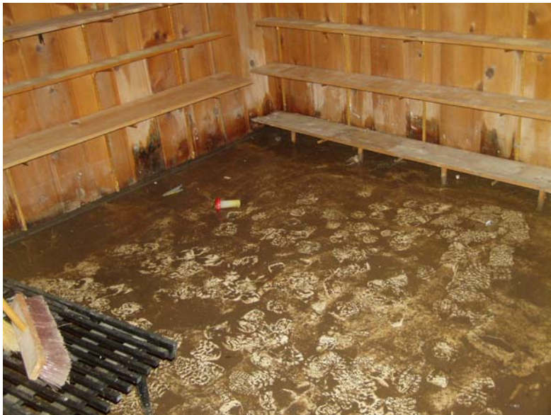
Extensive water seepage to basement.
