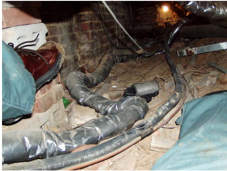
Crawl space - No vapor barrier on ground, loose ducts and wires on ground, trash and debris.
