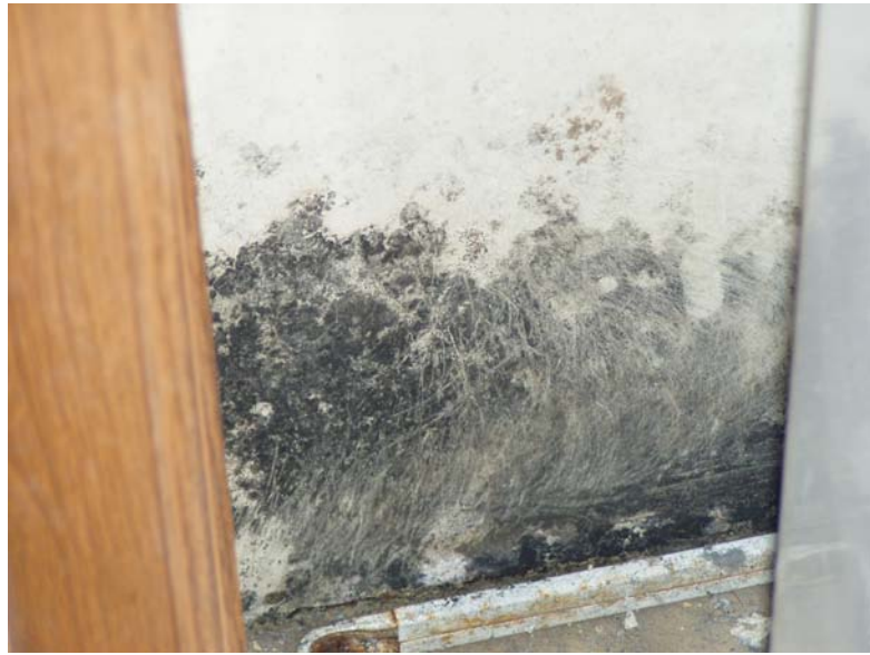
Mold growth on basement walls.(Unsafe)
