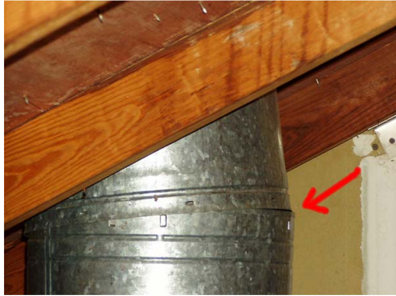
Metal fireplace flue separating. Attic view. (Unsafe)
