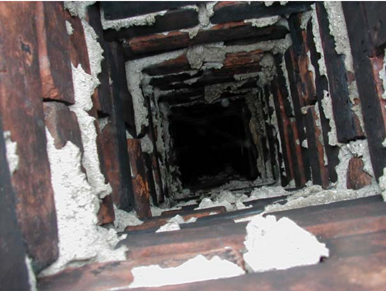
Old through-the-house chimney has no liner installed. (Unsafe)
