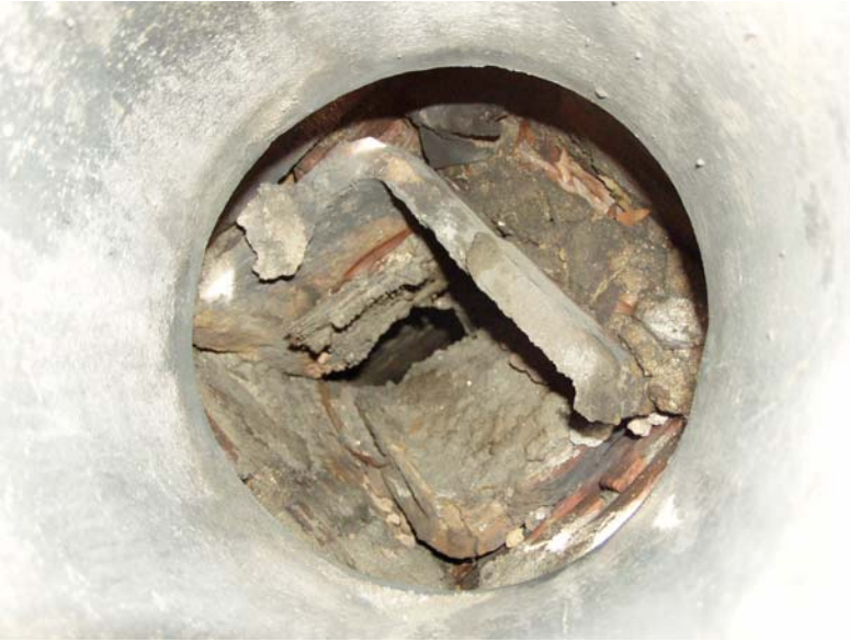
Failing flue liner, not safe for use.
