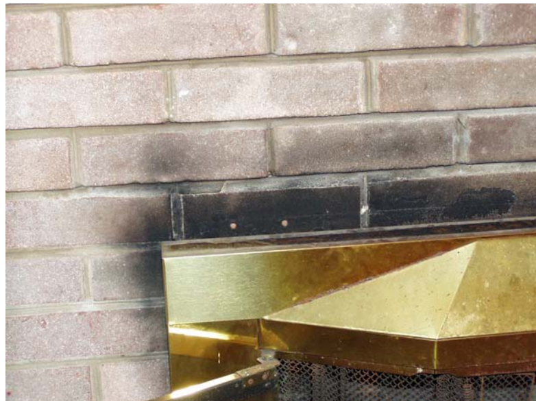
Smoke on fireplace face, due to poorly drafting chimney flue.
