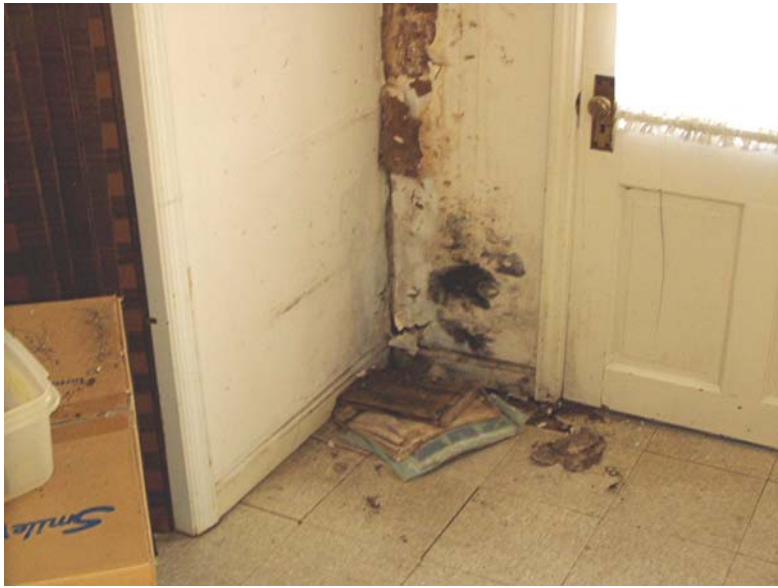
Leaking roof has caused rot damage to walls and mold growth. (safety)
