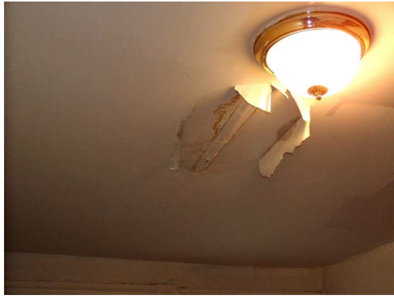
Bathroom plumbing leak is damaging kitchen ceiling.
